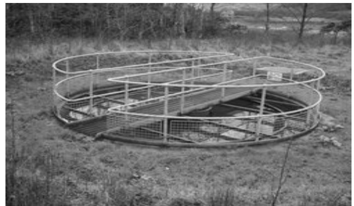
(B) Secondary sedimentation tank. Source: Wikipedia.
