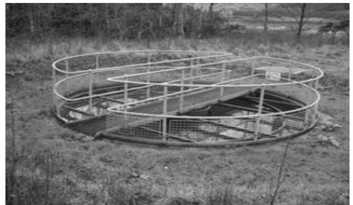
(B) Secondary sedimentation tank. Source: Wikipedia.
